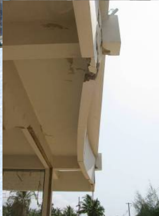
Lateral bending of beams
